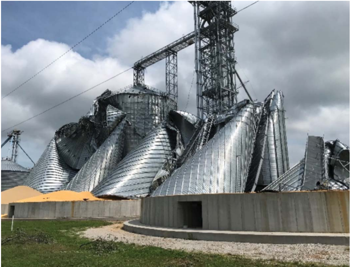
Grain bin damage from the August 10 derecho.
