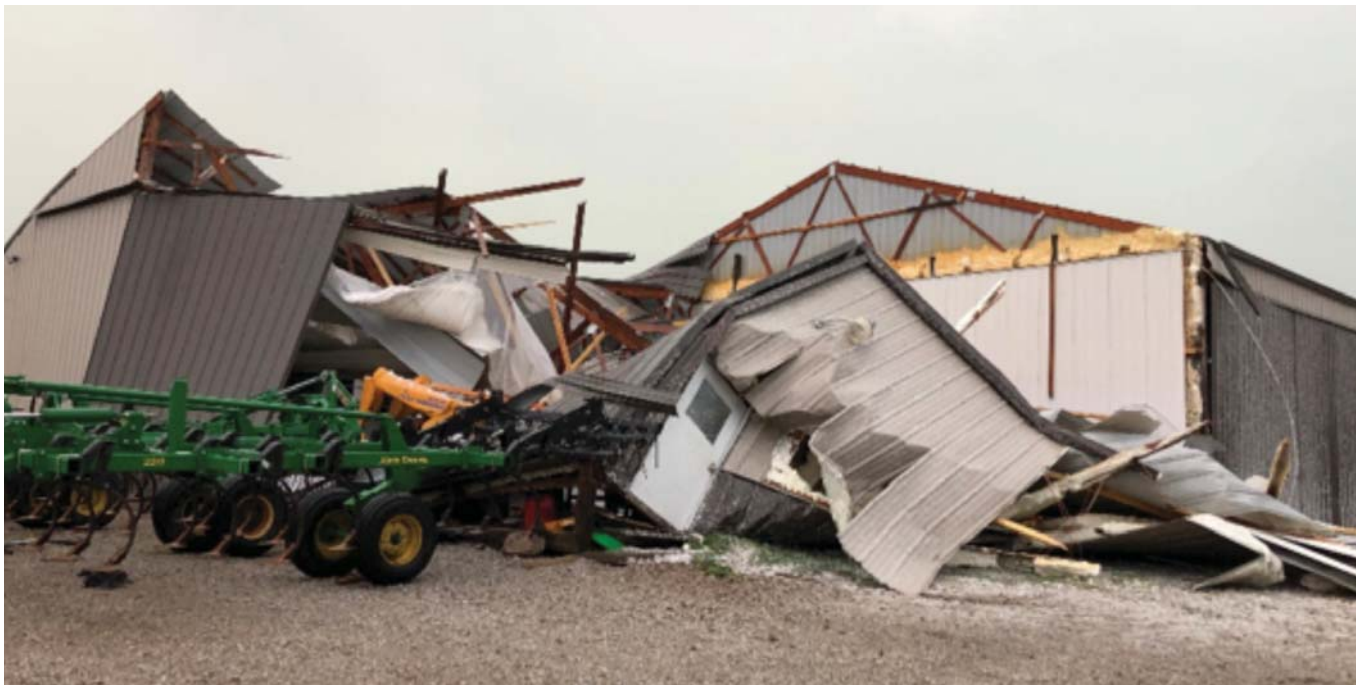
Building damage from the August 10 derecho.
